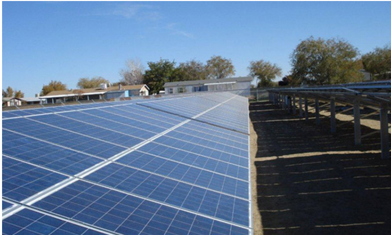
Figure 1. Desert Palms Mobile Home Park in Lancaster, CA was a project under the California Solar Initiative Multi-Family Affordable Solar Housing (MASH) Rebate Program. Photo credit: ZeroNet Energy Solutions
