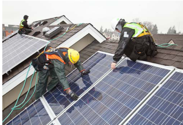
Figure 1. Solar panels being installed on public housing units. Photo: U.S. Department of Housing and Urban Development
